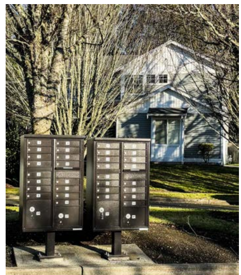
105 mailbox clusters were replaced in 2023 at a cost of $253,514. Five mailbox clusters were replaced in 2022 and 41 more will be replaced in 2024.
